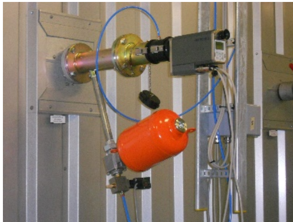
Figure 1: HEITRONICS solution installed on a boiler wall in a waste incineration plant
